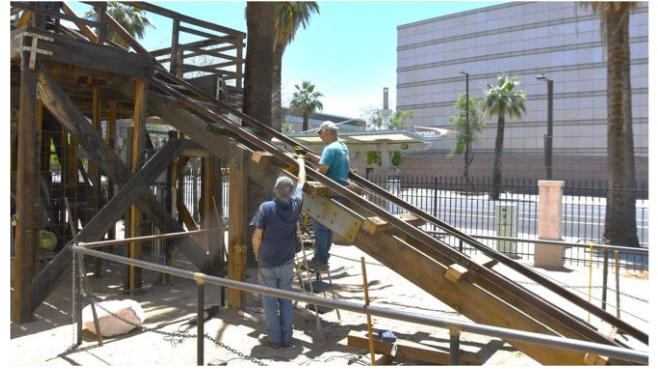
Don & Bill L. align a new timber on the incline. They did very well, replacing (5) of the cross ties. All of this was performed in 100° F weather.
