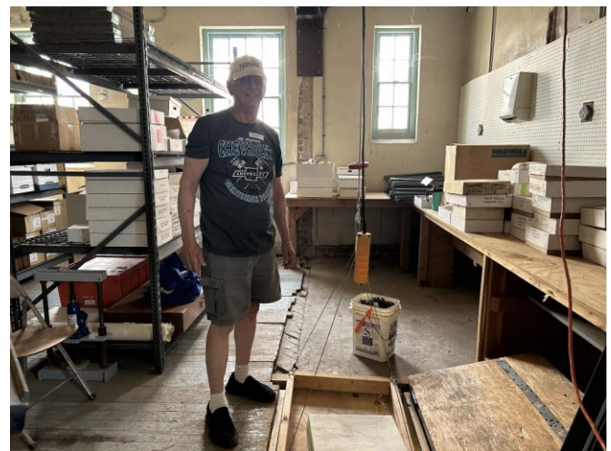
Club member Tom assisting with the winch that lifts heavy buckets directly up and out of the pit.
