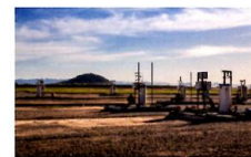
Florence Copper wellfield
