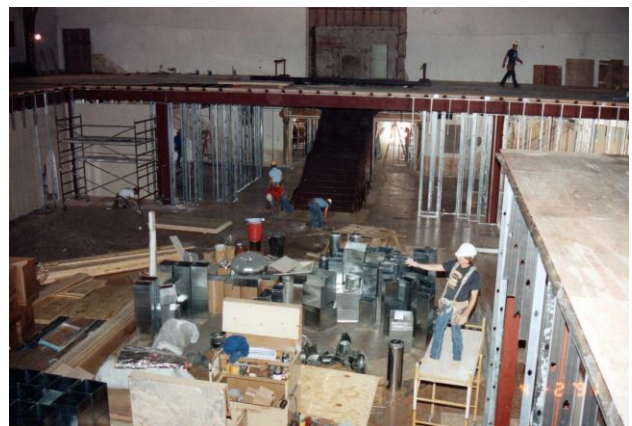
Another photo from the 1990 renovation with workers framing the mezzanine level of the main gallery.
