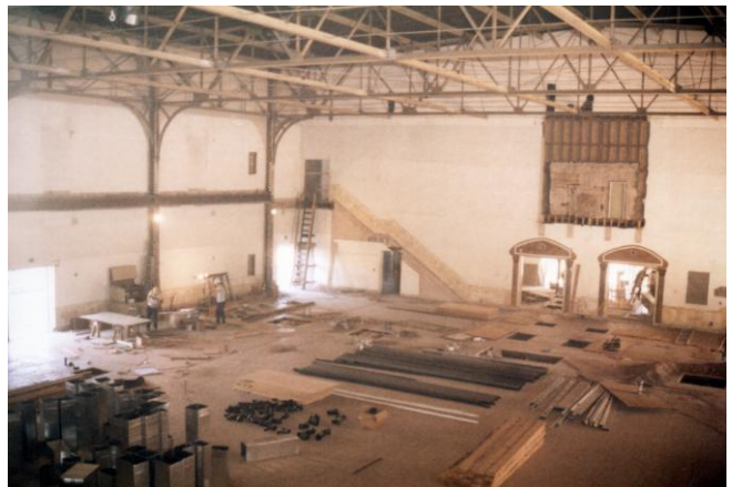
Photo from the 1990 renovation process showing work on the floor in the auditorium, later the museum's main gallery.
